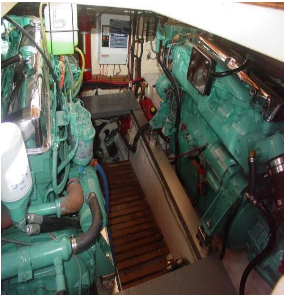
Typical Grand Banks 36 Engine Room Tight quarters in which to repair a motor, especially while underway in rough conditions, while ill.
